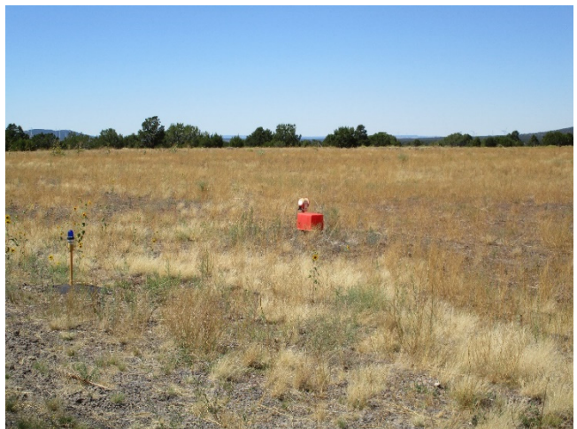
Runway End Identifier Lighting (REIL)
